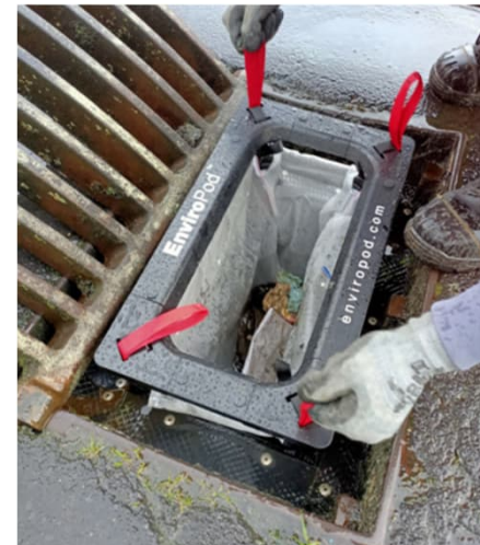
LittaTraps in Catchbasin
