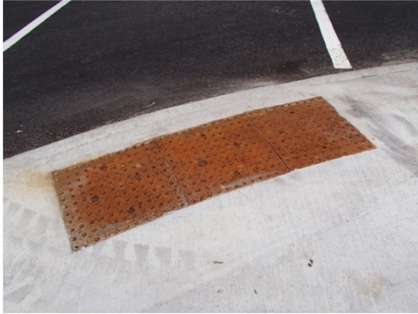
Exhibit 12: Tactile Walking Surface Indicator at Crosswalk
